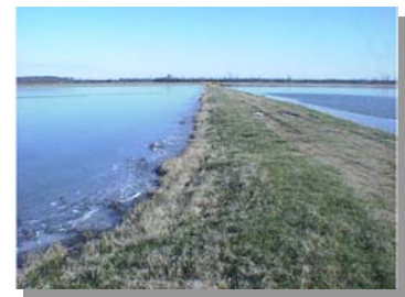
Embankment erosion by wind-wave action
